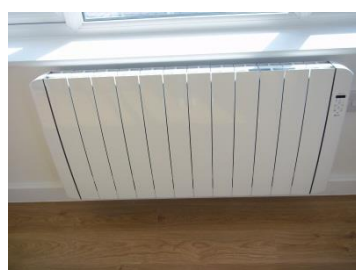
Electric wall heater
