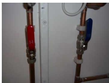
Water close off valves.
